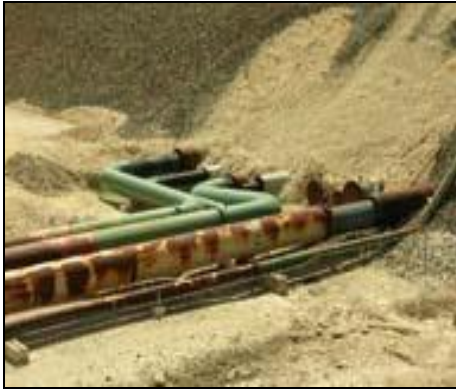
New Fuel Lines Side A
