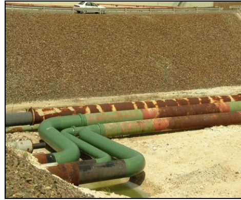
New Fuel Lines Side B
