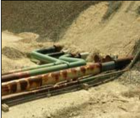
New Fuel Lines Side A
