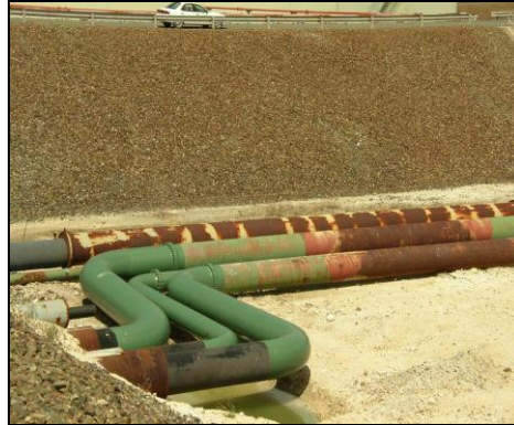
New Fuel Lines Side B
