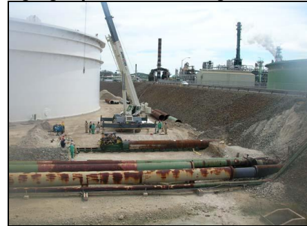
Aging Pipelines & 20' high dike
