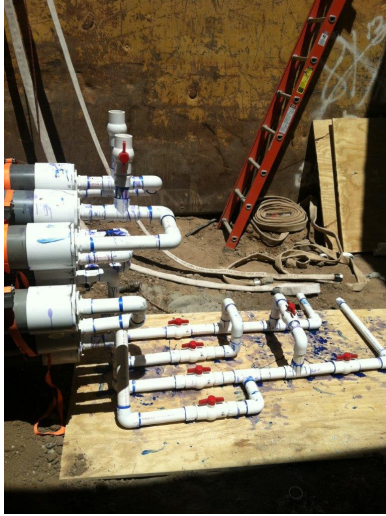
Figure 8: Plumbing on bore side
