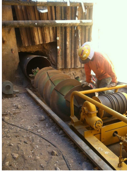
Figure 4: Hydraulic tugger being used to pull broken auger out of casing.
