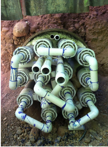
Figure 9: Plumbing on reception side 3 grout lines open in center
