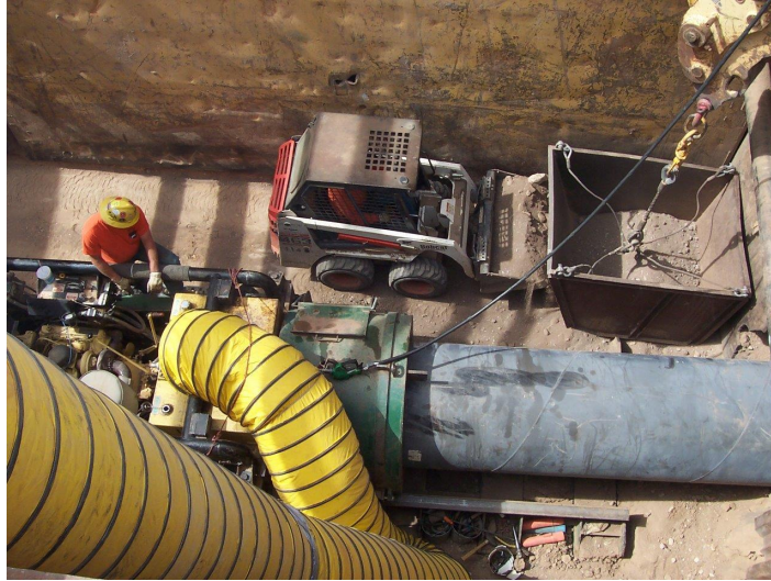
Figure 3: Bore Pit for Auger Bore Installation of 42” (106.7 cm) Steel Casing, with blower hooked up to help with cooling the machine.
